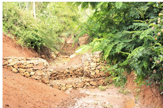
Figure 3: protected gully erosion in Ifa Jallela micro watershed
