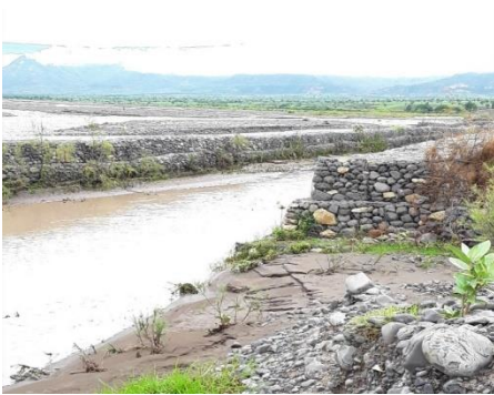
Figure 2. Secondary protection of sand filled gabion constriction to protect and save the land from Bersina river attack. 2021 GC
