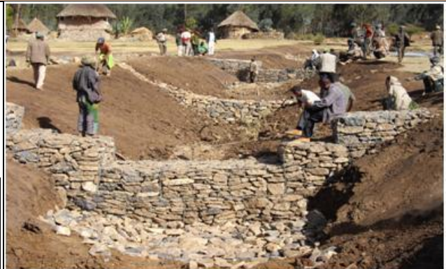
Fig 2. Gabion check-dam construction - stone filled, Amhara R., Farta Woreda, Alekt Wenz CW
