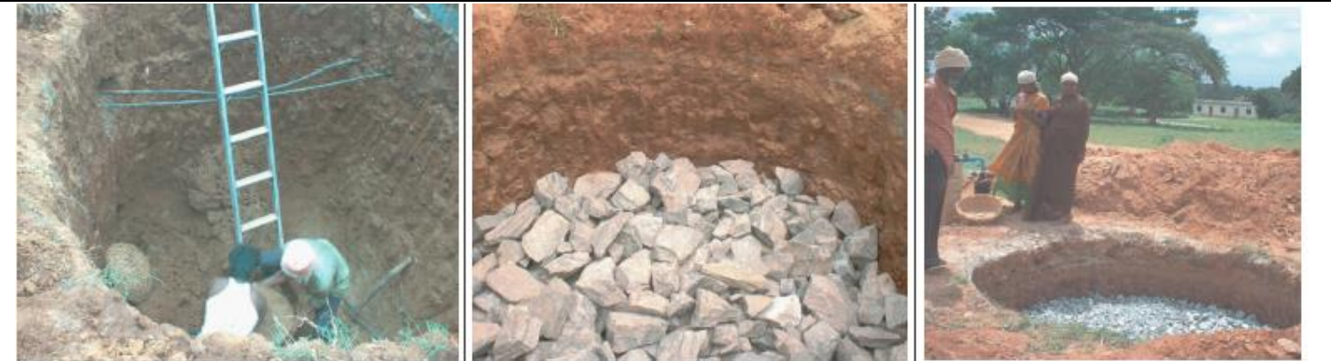
Fig 9. Excavation (left), backfilling with small stones and gravel (middle), and placement of coarse sand on top of the gravel
