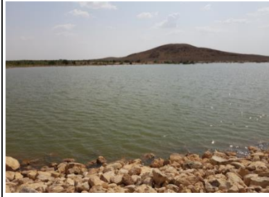
Fig 5. Scene of completed earthen dam, see the stone rip-rap on the upper side of the embankment
