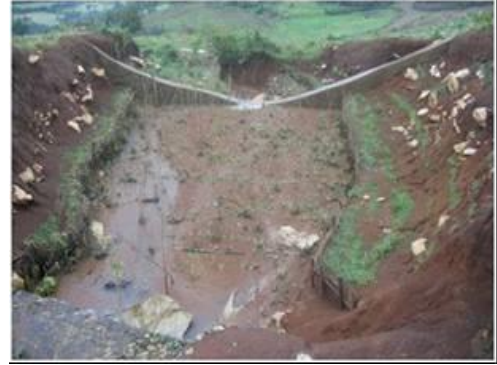
Fig 1. Arc-weir structure made up of cemented stone wall in horseshoe shape, Amhara R., Farta Woreda
