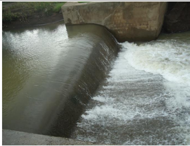
Fig 6. Closer look of a properly functioning diversion weir
