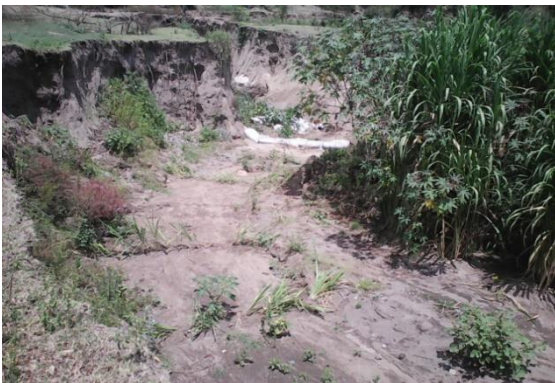
Figure 1 Gully erosion in Hawassa zuriya woreda at Fechena micro watershed in Obolodankaka kebele, 2015
