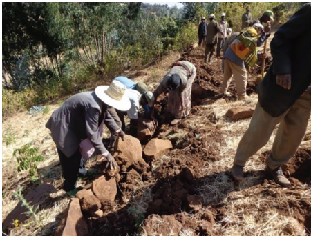
Figure 49: Community constructing hillside terrace on a communal hilly area (Ejere woreda, Oromia).
