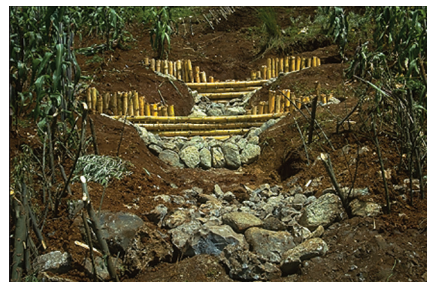
Figure 65: Debris retention and gully control structures with a notched weir to keep flow over the middle of the structure, scour protection added at each structure outlet and the structure is keyed into the firm soil banks.
