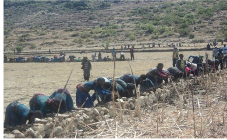
Figure 45: Community constructing stone-faced soil bund on hilly farmland (Wara Jarso woreda, Oromia).
