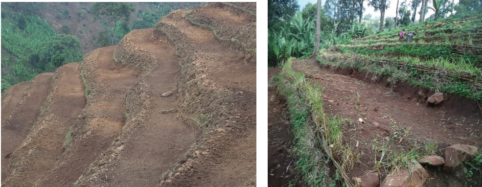
Figure 53: Bench terraces constructed on hilly individual land (Bore woreda, Oromia). Left: soil mixed with stone bench terrace. Right: bamboo bench terrace.
