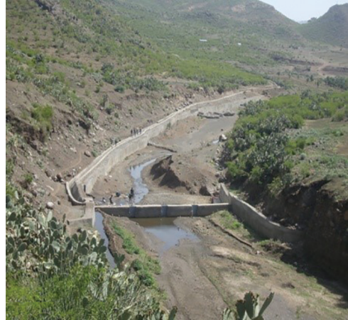
Figure 126: River diversion constructed by the community. Source: GIZ SLM archive, 2020 - Tigray region.
